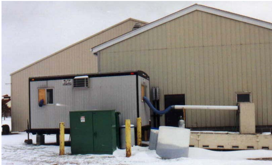
Figure 27. The photo of the field experimental system connected to manure tank.
