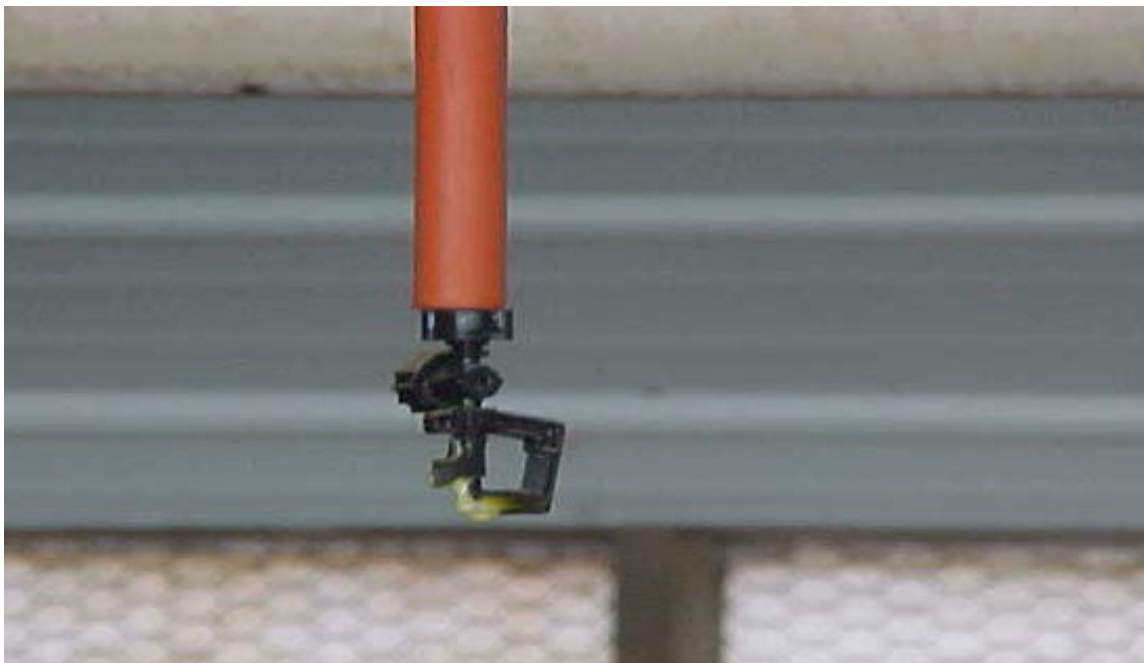
Figure 3. Spinner nozzle distributing oil-water mixture in finishing barn.
