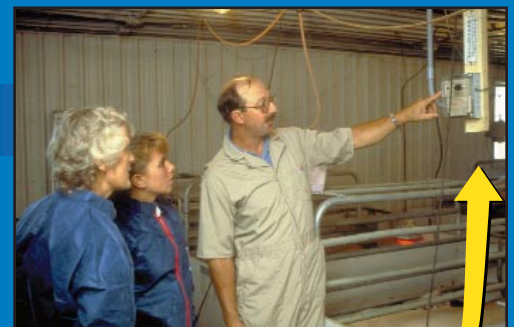
Temperature and fan control
